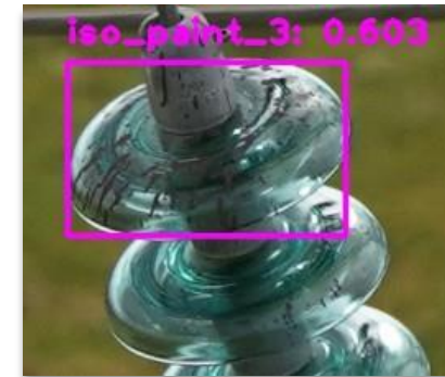
Paint on insulator
