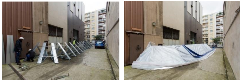
Cofferdams for Seine floods
